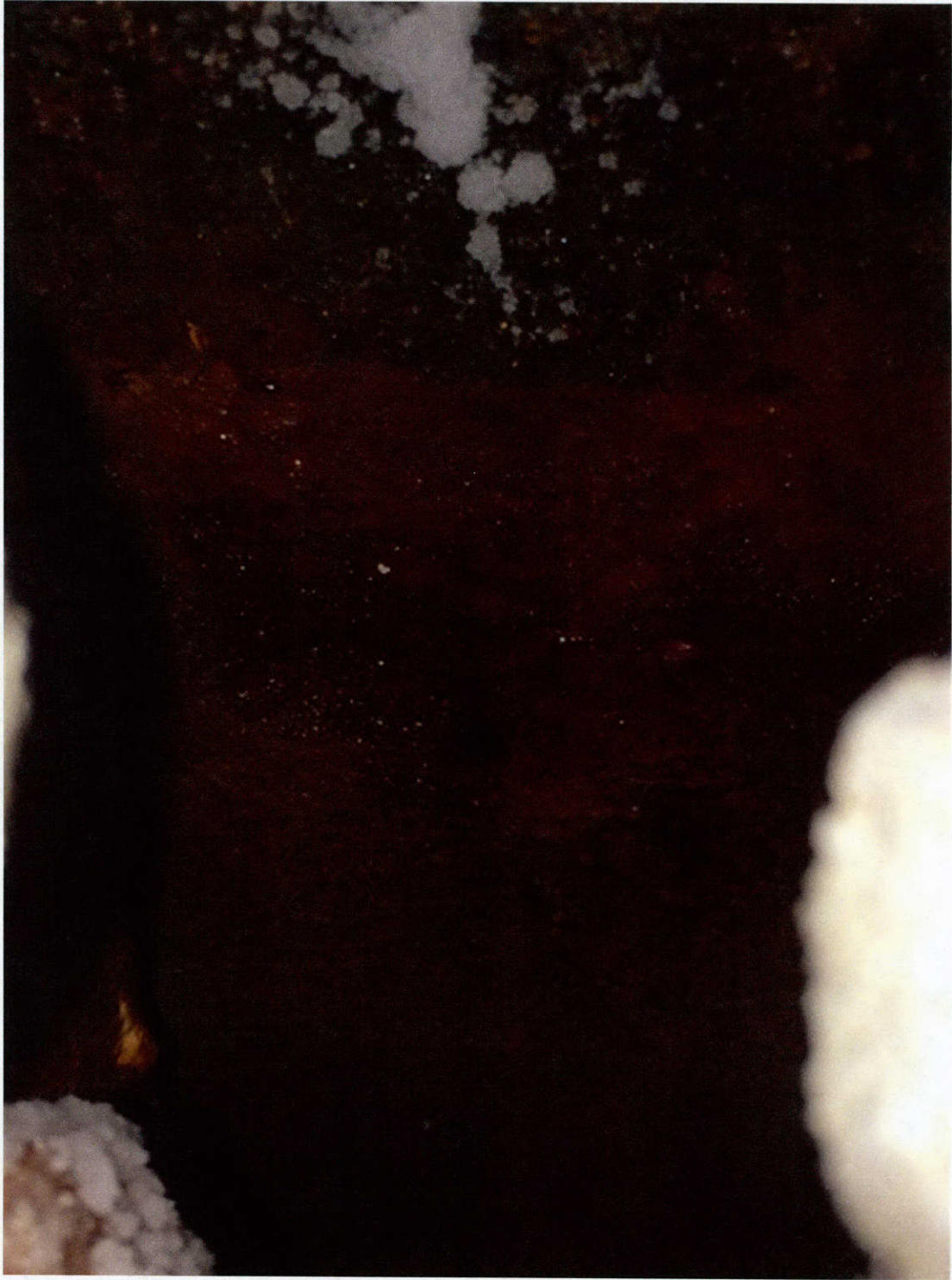
Figure 10.46: Web corrosion of Repair System 3 (S3-4-Cor)
