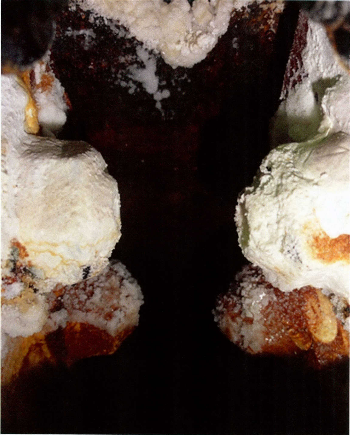
Figure 10.45: Bolt and web corrosion of Repair System 3 (S3-4-Cor)
