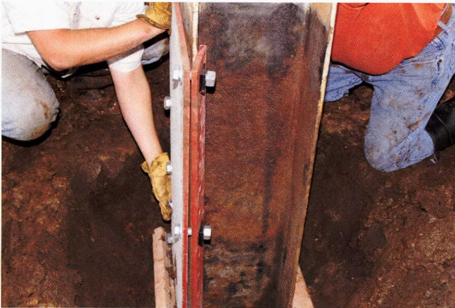
(b) Inside view
