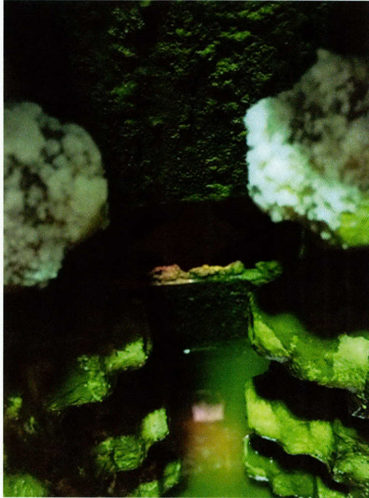
Figure 10.49: Web and bolt corrosion of Repair System 3 (S3-12-Cor)
