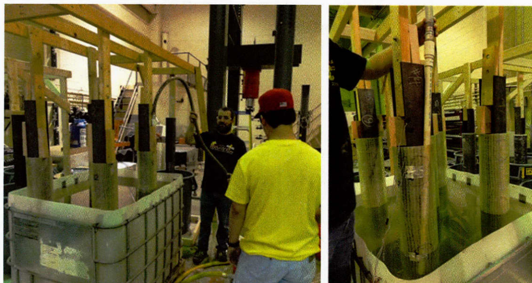
Figure 10.15: Grout injection into the voids between the GFRP shell and the pile
