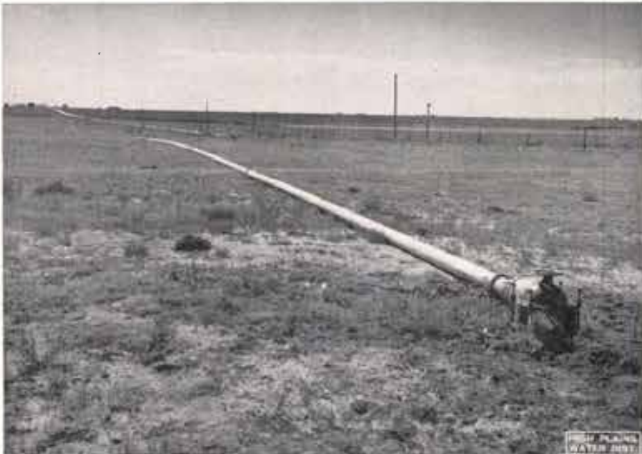
The picture above shows the 6-inch aluminum pipe that transports the lake water to a point on the King farm where it enters the permanent underground pipeline system. The hydrant shown is approximately 30 feet higher in elevation than the lake in the background.
