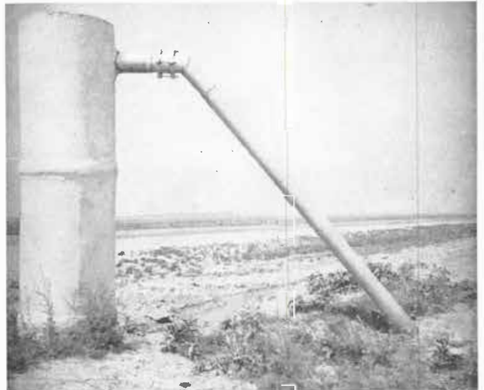
FIGURE 1. Pump discharge which lifts water higher than necessary and increases chances for mechanical damage to discharge pipe by tractors and machinery. The discharge could be below the ground surface.
