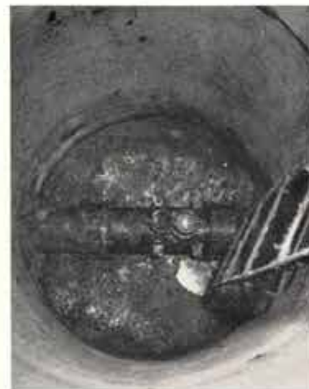
As the chemically-treated water gravity flows into the recharge well from the pit it passes through a flowmeter which records the number of gallons of water entering the underground aquifer.
