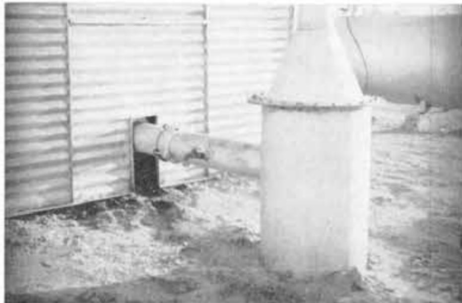
FIGURE 3. A good connection from pump to standpipe. Note straight discharge pipe with flexible coupling.
