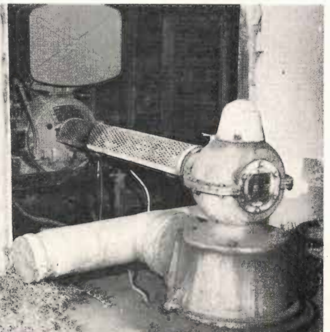
the pump. The shaft is covered in the picture on the right, minimizing the possibility of a person accidentally being injured by contact with the drive shaft.
