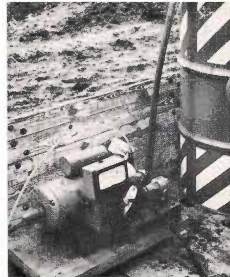
The flocculating chemical, mixed with water, is pumped from a steel drum through a plastic hose to the lake intake. The pump is driven by a small electric motor, which in turn is powered by a gasoline motor generator.
