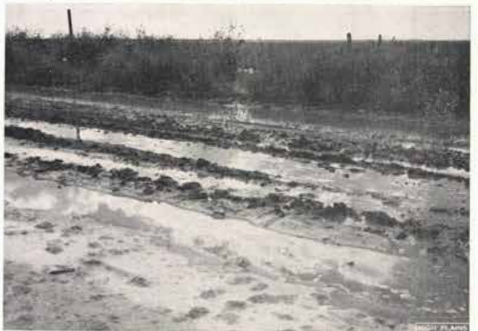
Above is pictured a county road in the southern High Plains which has been completely inundated by agricultural "tail-water." This is not only a nuisance and a waste but also a hazard to the safety of persons who might be driving on this road. The picture was taken during the early part of September 1959.
