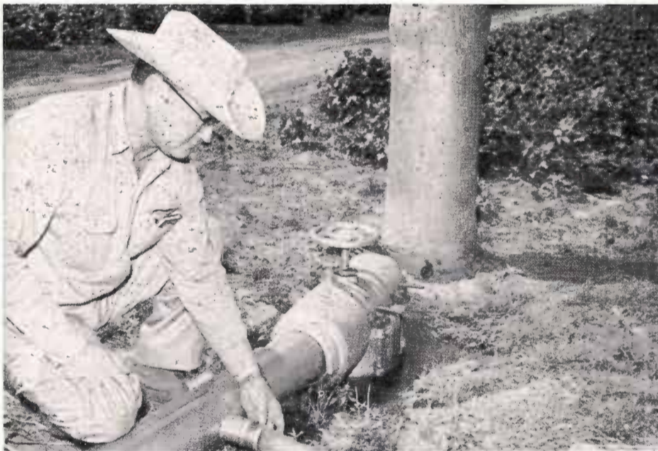
Irrigation water is pumped from the wells on the Unfred farm to the growing crops through a system of underground pipe lines. Outlets are spaced over the farm through which irrigation water may be transferred to the surface at any time.
