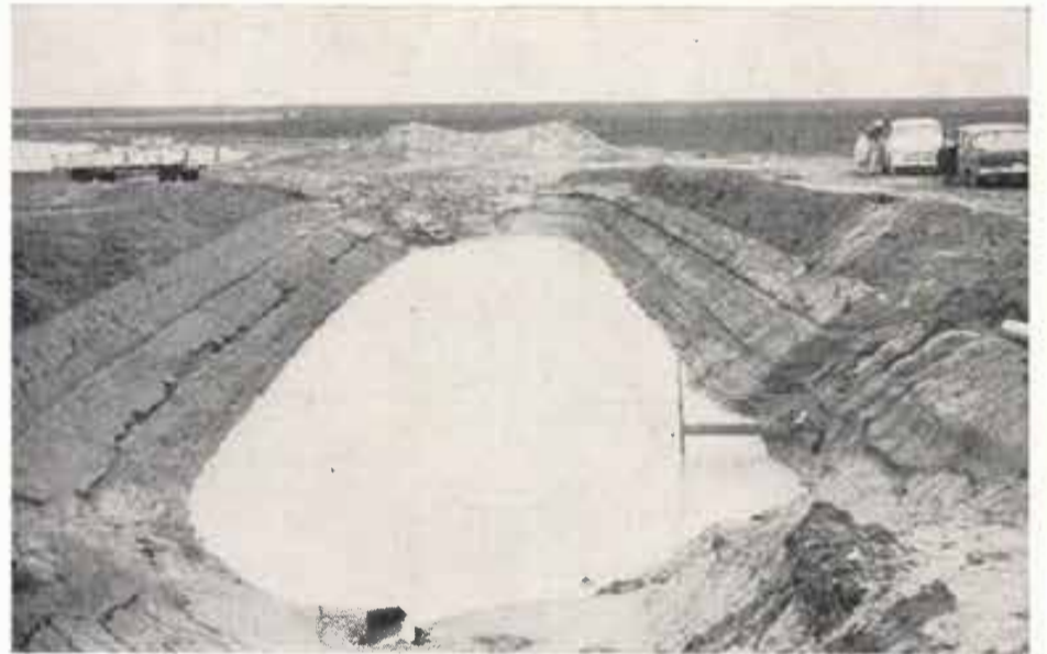
FIGURE 4—View of Sutton Lake and settling sump. Chemical in solution form was mixed with lake water using equipment on trailer shown at left.
