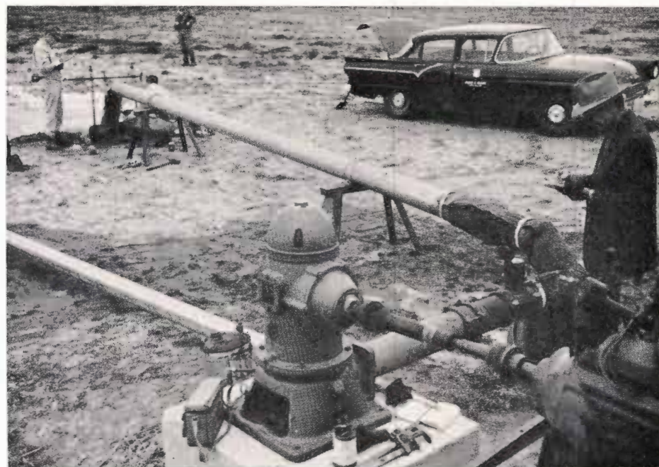
Pictured, in the foreground above, is the Moreland recharge well. You will note the sampling device installed at the discharge end of the aluminum pipe. Also, note the flow-meter installed in the discharge line near the pump base.
