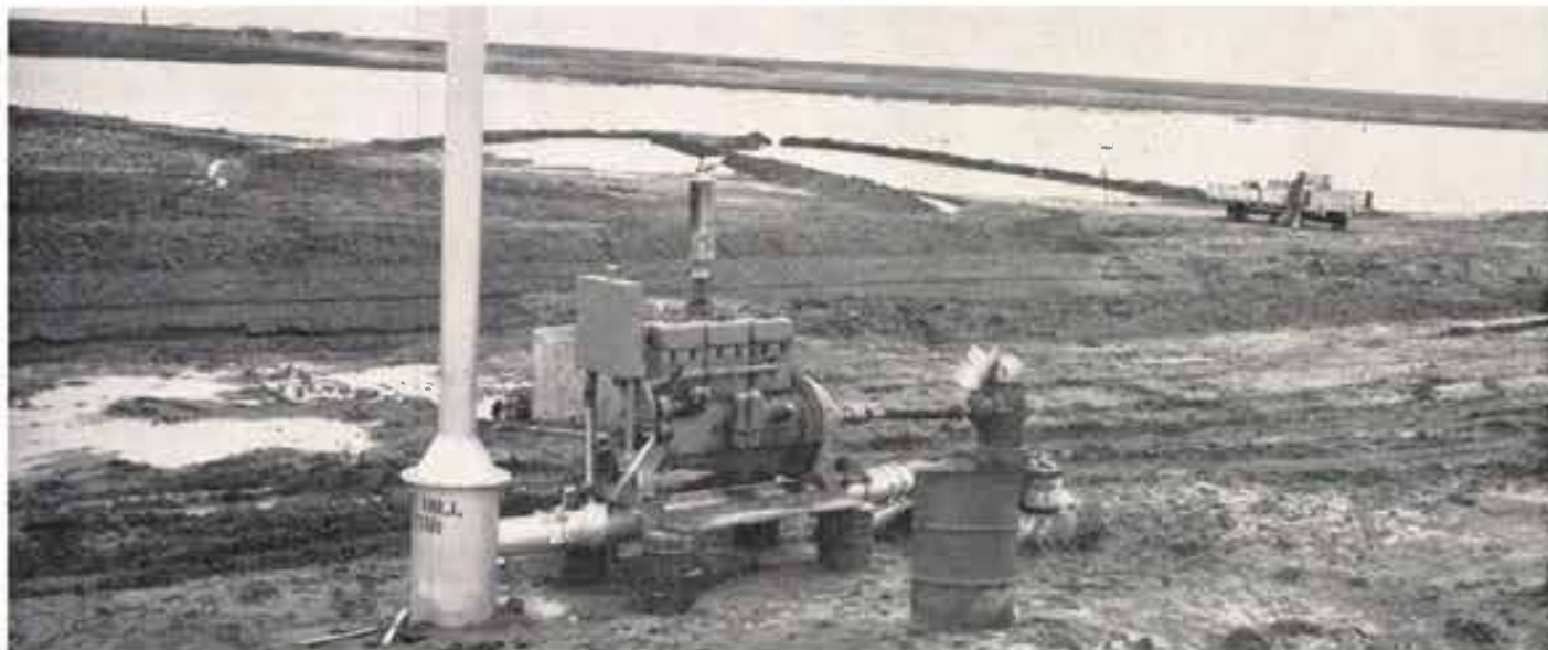
The picture above shows an overall view of the Bill Sutton lake and recharge well. Lake water drains by gravity into a concrete pipeline. The flocculating chemical is injected at the lake intake. The chemical and lake water mix thoroughly in the pipeline between the lake and a large earthen pit. The
