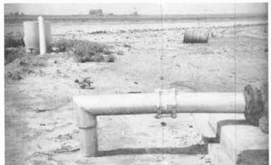
FIGURE 2. Sharp bend (foreground) increases horsepower required for pumping. Discharge pipe (background) lifts water higher than necessary.
