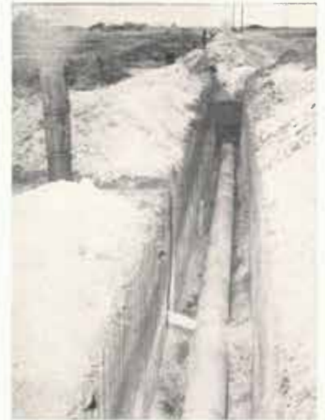
A segment of the system's main line is shown above. Note the lateral line connection near the bottom of the picture. Water that enters the main line from the lateral line may be metered through the riser shown at the left.
