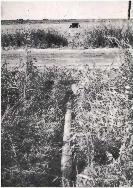
Water is pumped to growing crops from the lake through 6-inch aluminum pipe under the paved road through a metal culvert.
