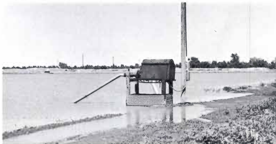
Tommy McKinnon equipped the lake with this centrifugal pump driven by a 30-horsepower electric motor. It will pump 650-700 gallons per minute.
