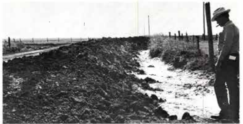
Large mounds of silt removed from bar ditches by Deaf Smith County road maintenance crews are piled along county roads. (See story on page 1.)
