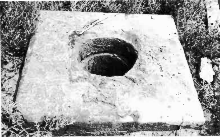
This is an open abandoned well. Note the size of the hole. It would be very easy for a fully grown person to fall into it.
