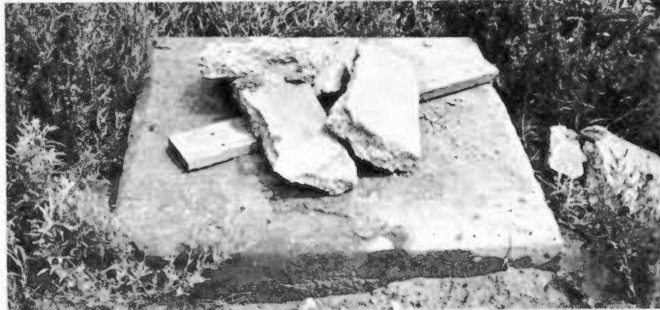
This is an example of an incorrect way to cap a well. The boards and rocks are light enough in weight for a child to lift, leaving the hole open.
