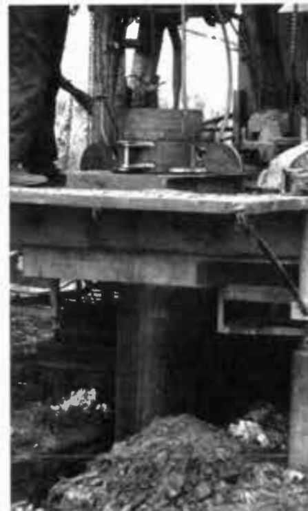
LOWERING THE SCREEN —Drillers, L. K. Howard and Sons, install the new Johnson Agri-Screen into a well near Clovis, New Mexico. The screen slides into the hole with ease and obviously presents no additional concerns for the driller.
