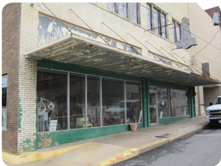
(Top) 134 1st St. SW building in Paris before paint removal; (middle) single layer of paint on upper façade; (bottom) multiple layers of paint on the lower façade.
