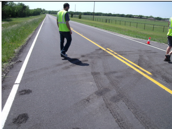
Tear marks (bottom left) from power to rear tires damaging the microsurfacing. The microsurfacing was still slightly soft when visited 5-6 months after construction. Demonstrates importance of creating an adequate mix design to ensure proper curing.
