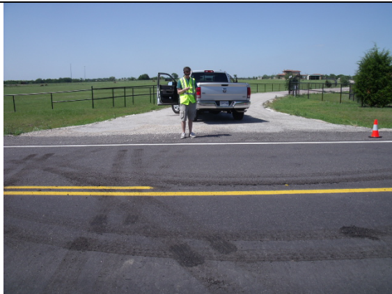
Damage to intersection most likely from early opening to traffic.
